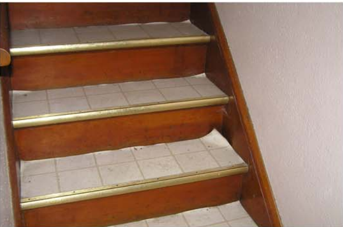
Before: Orfield-Skrivseth recommended refinishing the old stairs. "Refinishing old stairs is huge, because they are a psychological transition space," she says. "If they're dirty and peeling then you don't want to walk on it or see where they lead, but when they're nice and clean then people want to see where the stairs go."
