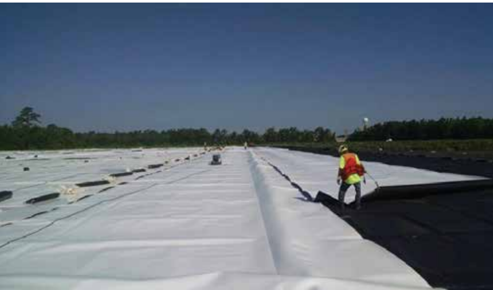
PHOTO 2 The geogrid was installed to distribute surface loads across a wider area.
