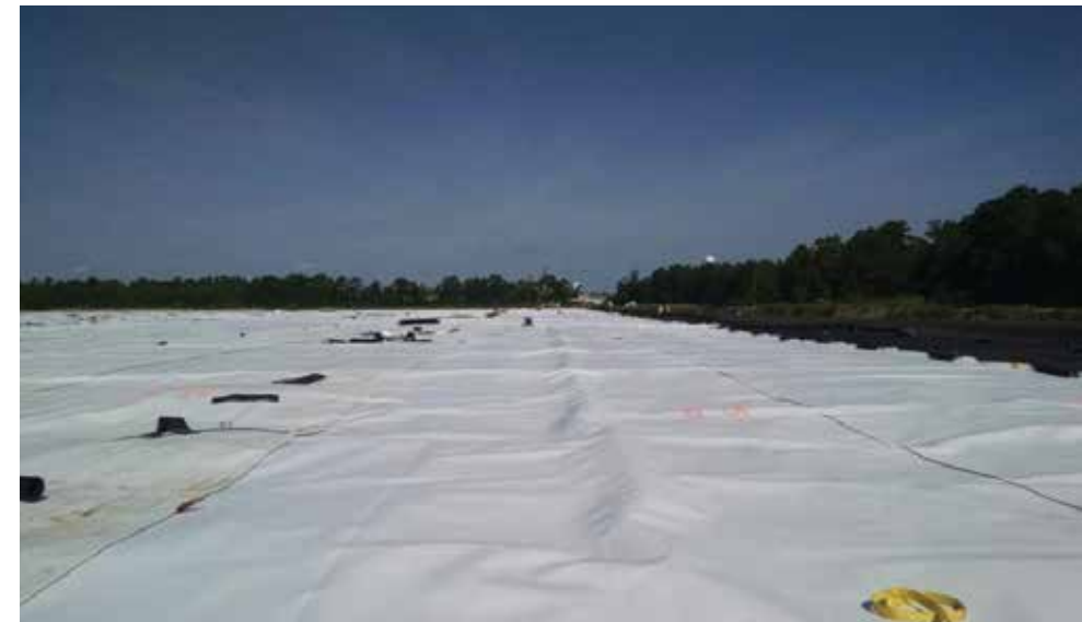
PHOTO 3 A white 80-mil HDPE geomembrane was installed, stretching across the entire 12-acre basin.
