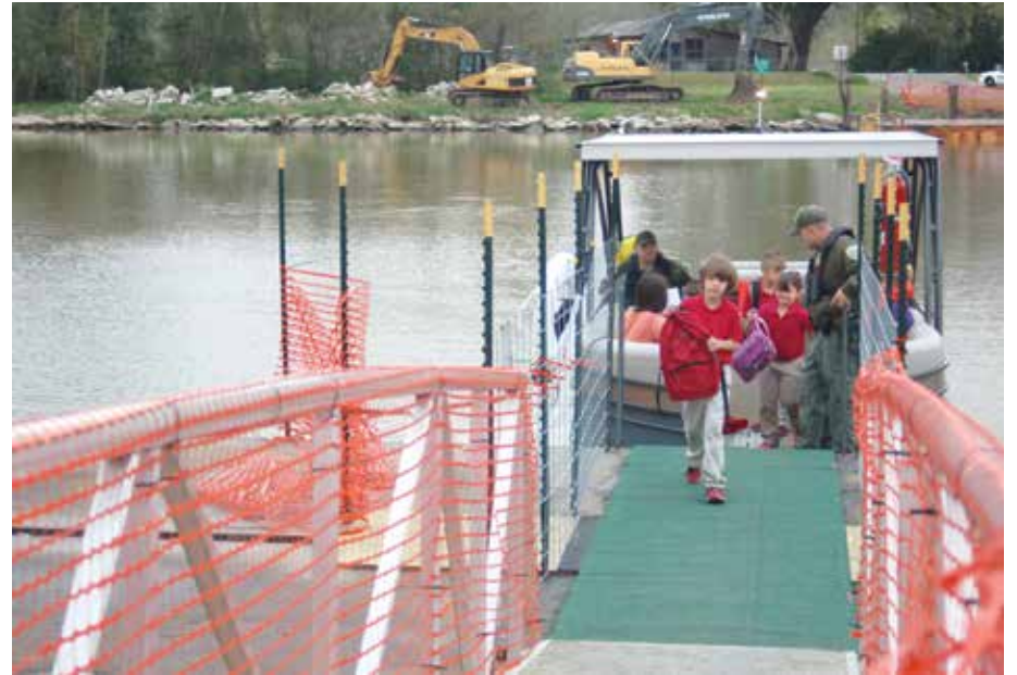
Students disembark from the pontoon boat transporting them across the Intracoastal Waterway. Shown in the background are La. Department of Wildlife and Fisheries agents who operate the pedestrian crossing service while the bridge is being repaired.
