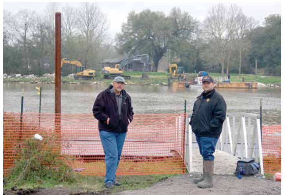
Parish President J. Mitchell Ourso, Jr. and Sheriff Brett Stassi inspect work at the site of the temporary pedestrian crossing service they initiated to help local residents get across the waterway for the approximately three months of bridge repairs.
