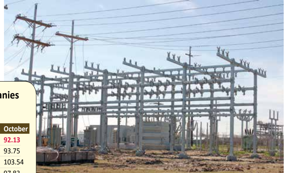
The city's new transformer, scheduled to be running by this summer, will make the electrical system more reliable. Shown above are new transmission lines for the transformer.
